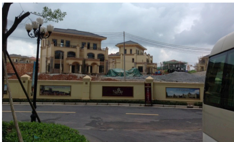
Evergrande Springs Metropolis in Enping, Guangdong. Above: the sales office. Below: villas under construction. Planned for the site are an exhibition center, a “food street” with food from eight countries and a hotel. There will be 16,785 housing units. The greater Enping region has a population of only a few thousand. The city of Jiangmen is about three hours away by car and Foshan about two hours. Photos by J Capital | June 2014.
